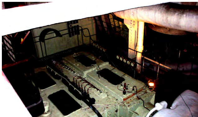
A view of the engine room aboard the Queen Mary
